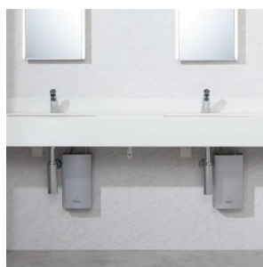
INAX's water heating hands-free faucets in Japan supplies the right amount of water at the appropriate temperature in public bathrooms.
