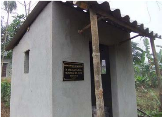
A toilet constructed by villagers. On the plate are the year of construction and LIXIL’s financial contribution to the construction costs.
