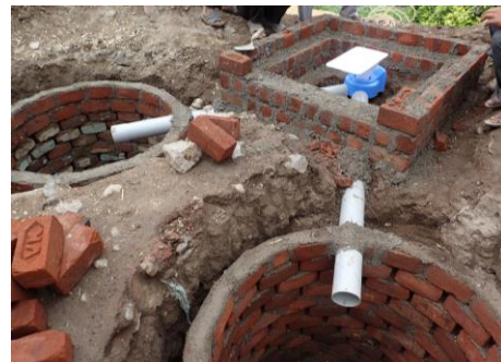
SATO's new V-Trap connection system, a twin-pit pour-flush latrine, being installed by local masons
