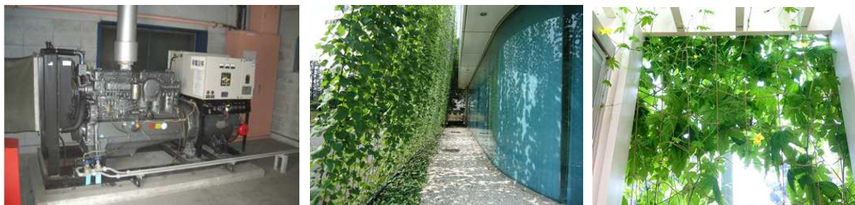
▲ Tsukuba Factory: emergency generator for water supply
